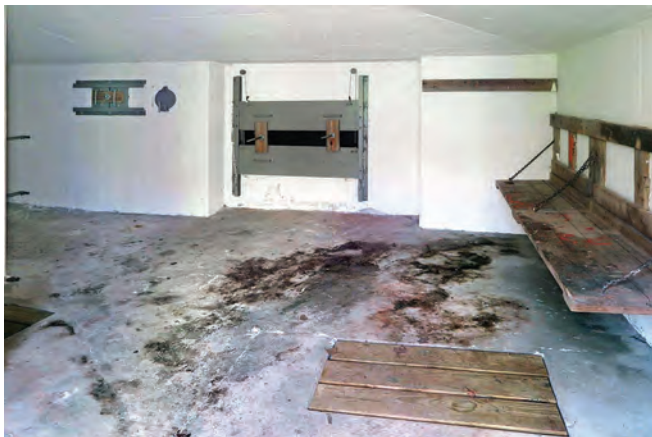
Main firing loop in the anti-tank pill box; a smaller loophole on the left can also be seen. The wooden planking on the floor covers recesses which would have held the gun's split trail to reduce recoil
